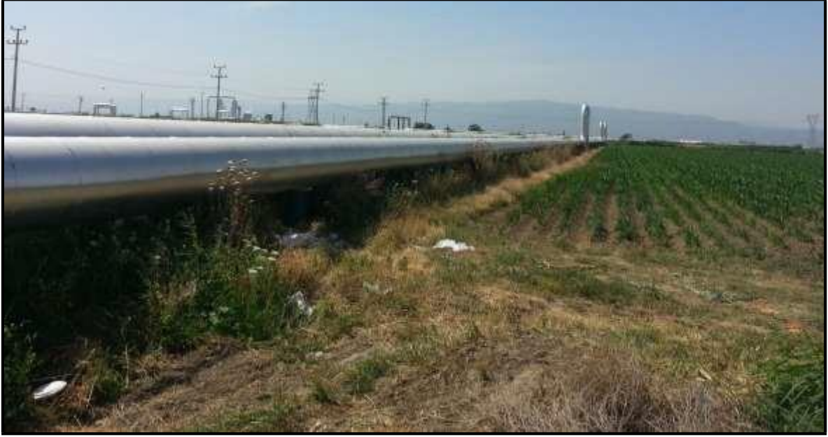
Figure 94. View of the existing piping system
