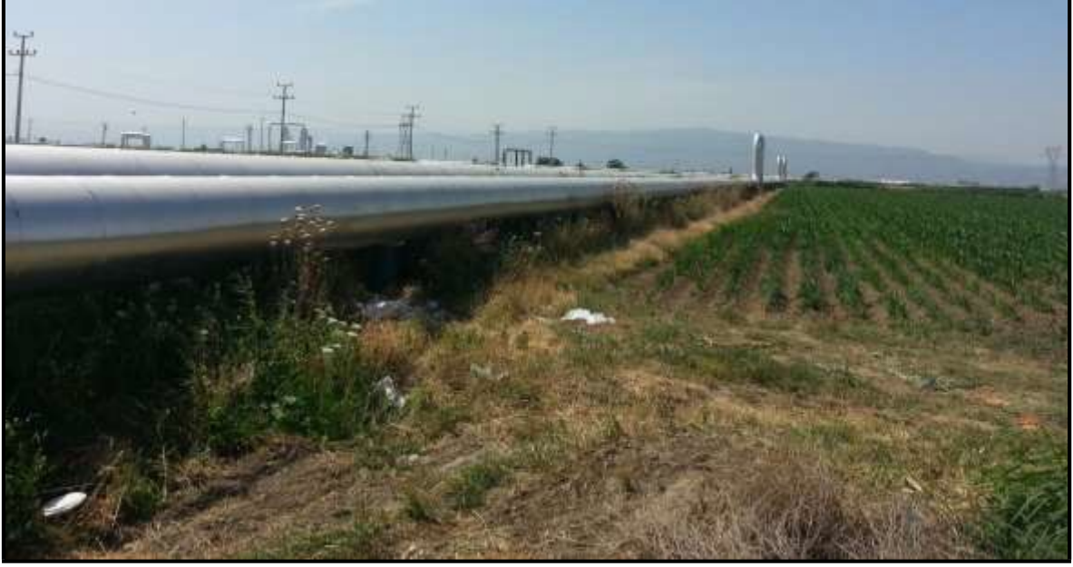
Figure 95. View of the Existing Piping System
